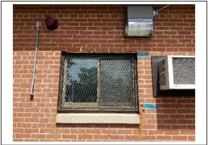
2. Sample locations 073018C01 (south side, west window, top header) and 073018M02 (masonry)
