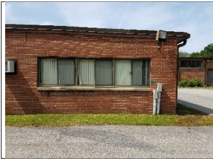
7. Sample location 073018C09 (east side, north window, side trim)
